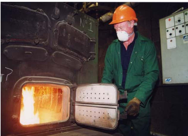
Terry, the caretaker, demonstrates the school's wood pellet boiler
