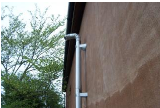
The Flue for the Pellet Stove
