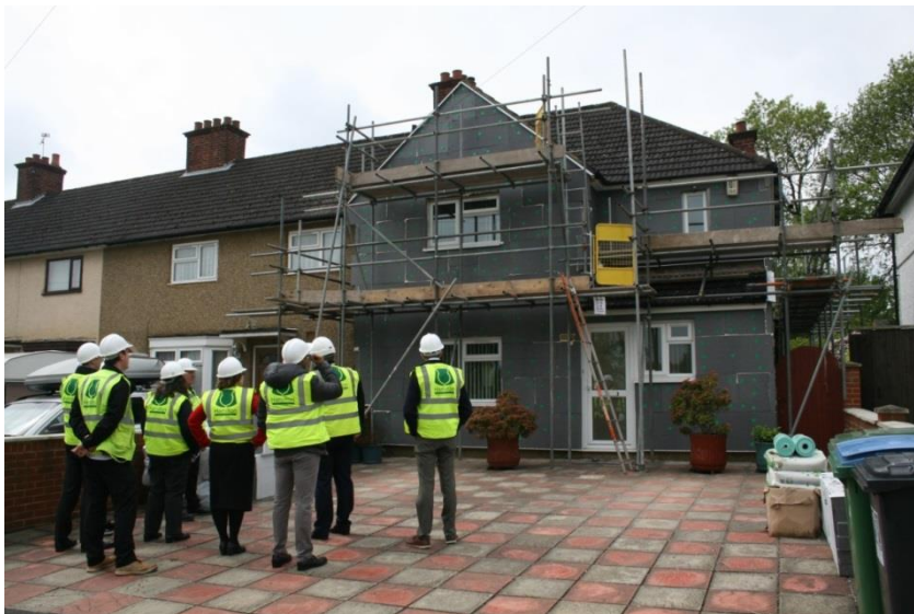
©National Energy Foundation – viewing EWI in progress with Hamilton (Building Contractors) Ltd
